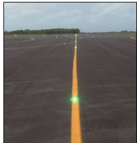
Green Taxiway Centreline Lights
