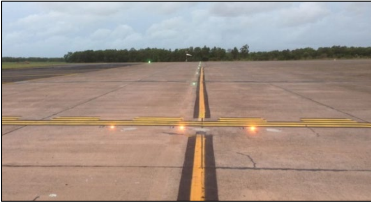
RWY Holding Position Lights
