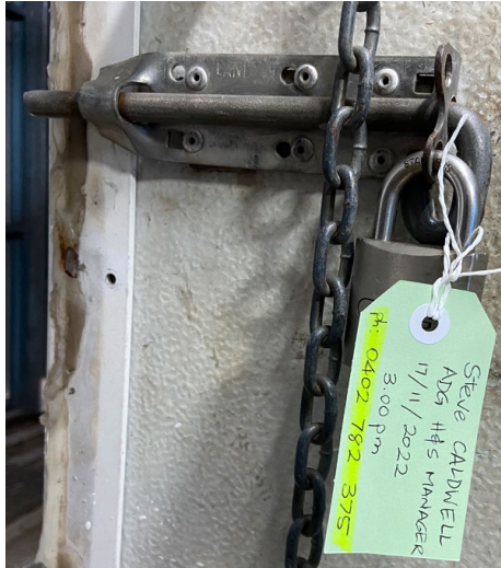
Photo 1 – Terminal roof access door is locked in the open position when you access the roof
