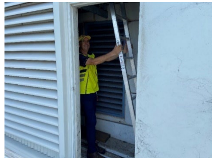
Photo 6.30 – Area Central PR filter – Correct ladder discipline
