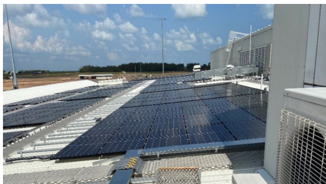
Photo 4.5 – Burn hazard and cut hazard – When walking & working near solar panels workers must wear gloves
