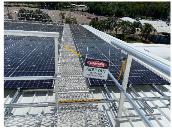
Photo 6.13– Area B West – Prohibited access to eastern sloping walkway from top walkway – Must have a Working at Height Permit approved by ADG Health & Safety Manager or approved delegate.
