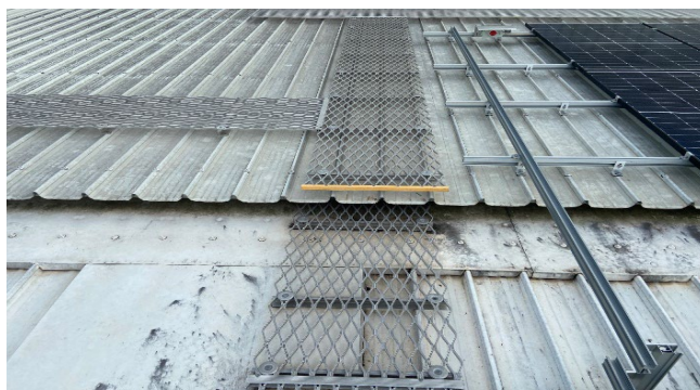
Photo 4.4 – Trip hazards (Change of height) – highlighted or marked with strip
