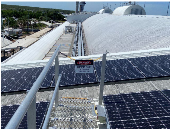
Photo 6.12 – Area B West – Prohibited access to eastern sloping walkway from bottom walkway– Must have a Working at Height Permit approved by ADG Health & Safety Manager or approved delegate.
