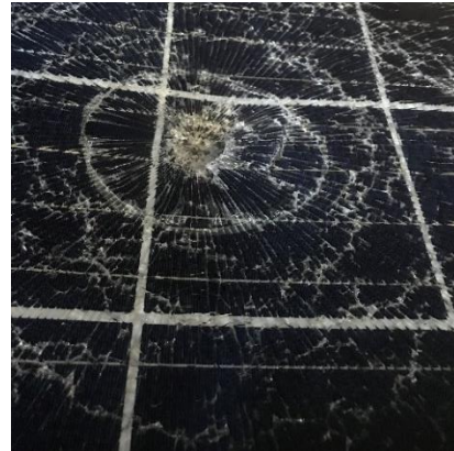
Damage to solar panel from door
