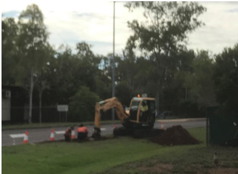
Worker near operating digger bucket not wearing a hard hat
