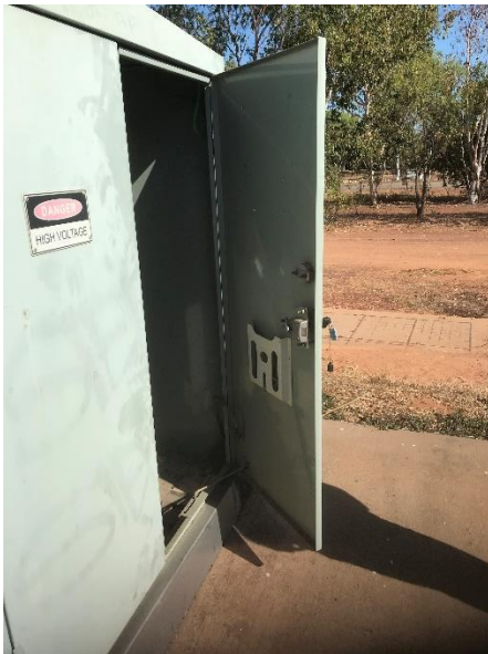
Sub 26 – where doors were found to be open
