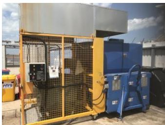
Compactable waste - All staff using the compactor must be trained in the use of the compactor
